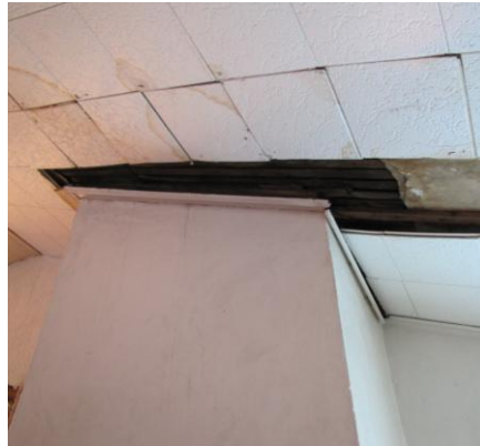
AME Zion Church second floor balcony water damage from Hurricane Sandy (2012).
