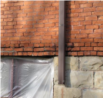
AME Zion Church exterior bricks in need of repointing.
