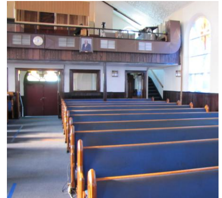
AME Zion Church second floor balcony. Water damage near the top of the photo in the center.
